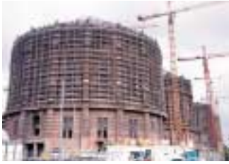
High-rises are being built in the cylinders of the largest Gasometer compound in Europe.
